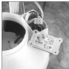
Romex wiring – Top View
