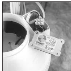
Romex wiring - Top View
